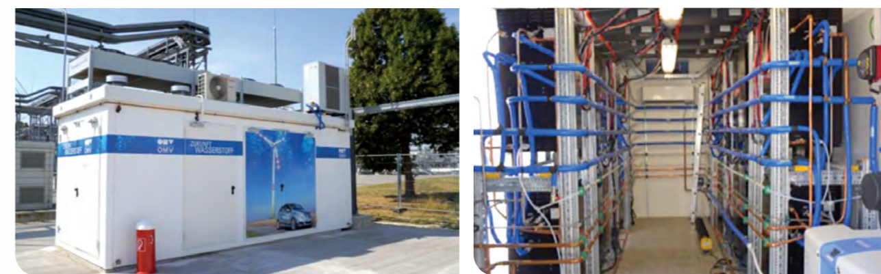
Figure 4: Project Wind2Hydrogen with electrolyse plant (left) and periphery (right)
