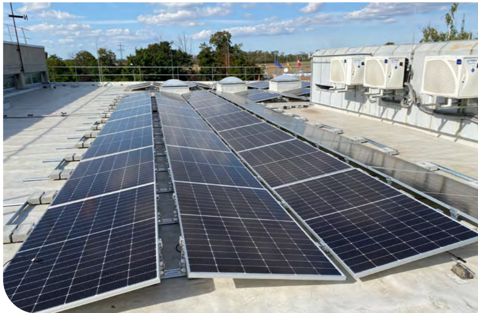
Figure 3: Rooftop installation of n-type PV modules in two orientations: SE and NW.
