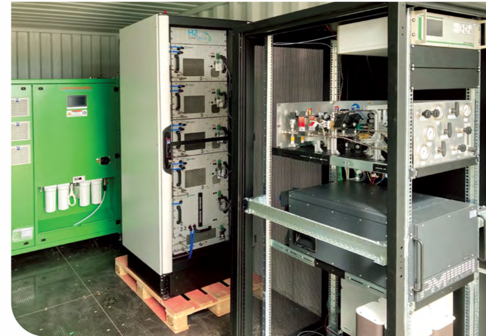
Figure 5: Main components of the P2P H 2 -Demonstrator, from left to right: PEM electrolyser, AEM electrolyser and cabinet with gas monitoring, measurement and control unit and fuel cell (from top to bottom).
